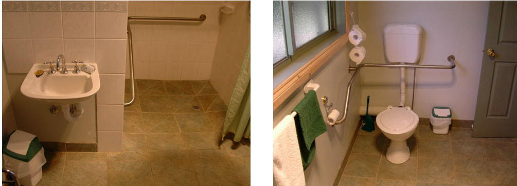
Pictures 8 & 9. Shower and toilet
